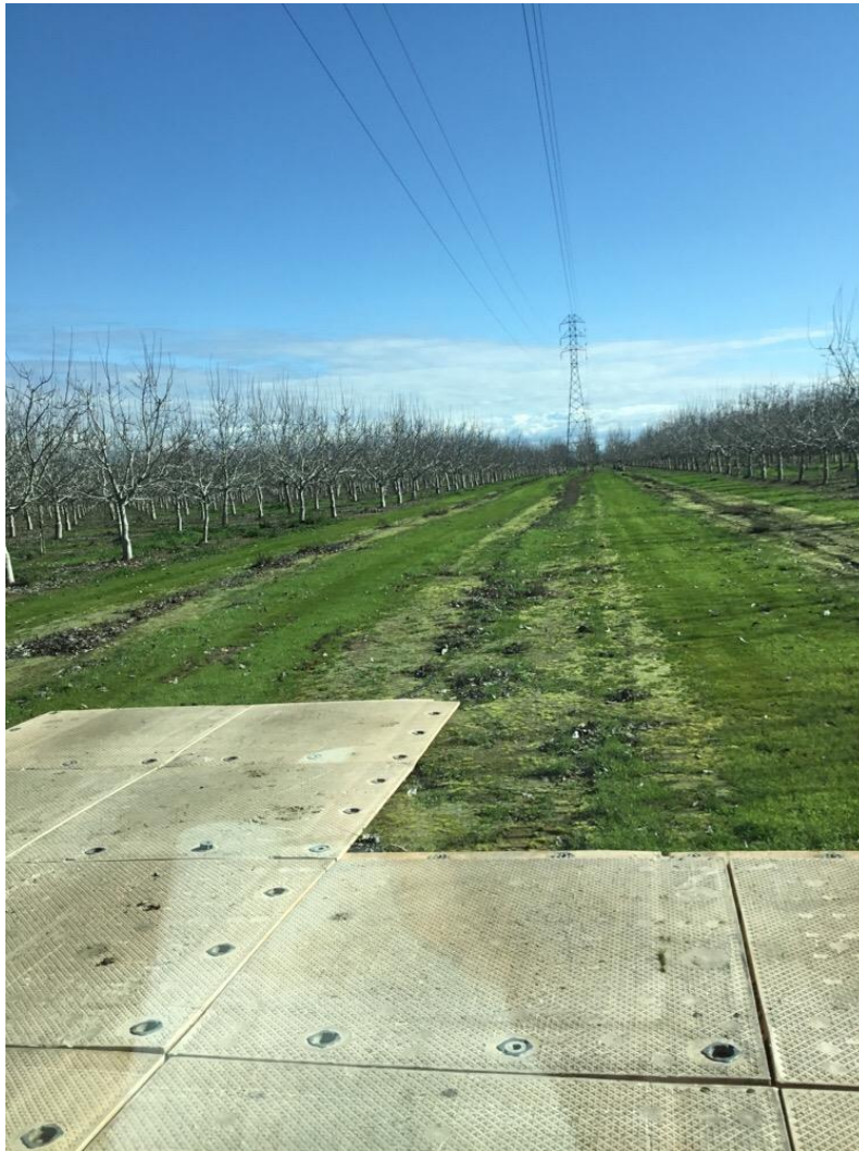
Photo 3: Mats installed to prevent track-out at structure 5/25, in accordance with APM HYDRO-1.
