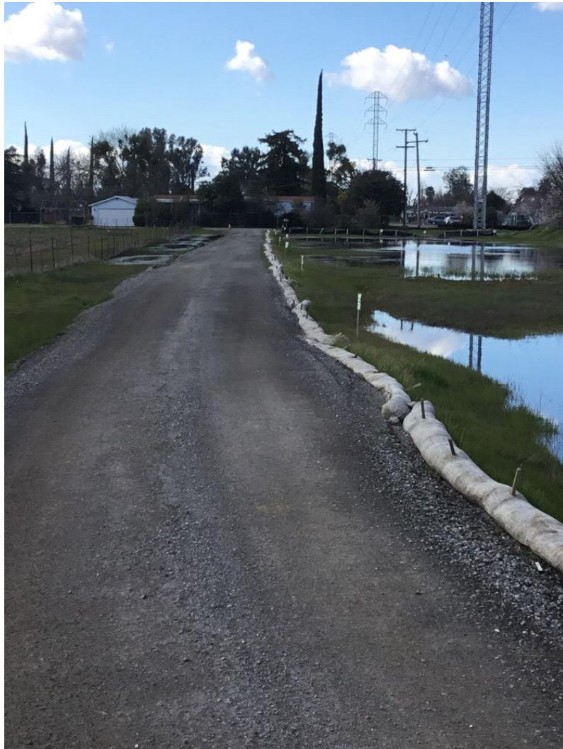
Photo 4: Wattles along the access road to PS 0/1B were observed to be intact and in good condition, in accordance with APM HYDRO-1.
