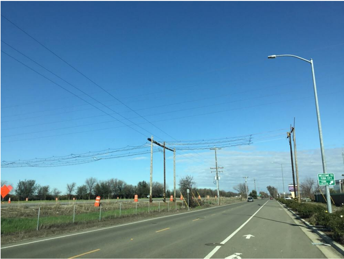
Photo 1: CPUC EM observed installed netting to protect Hwy 99 during wire pulling activities.
